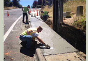
Sidewalks are an important component of the walking route to school. In some cases, a pathway (or designated walkway) can be implemented instead of a full sidewalk.
