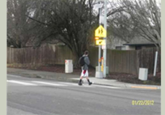
A RRFB is an active warning device used to alert motorists of crossing pedestrians. They remain dark until activated by pedestrians.
